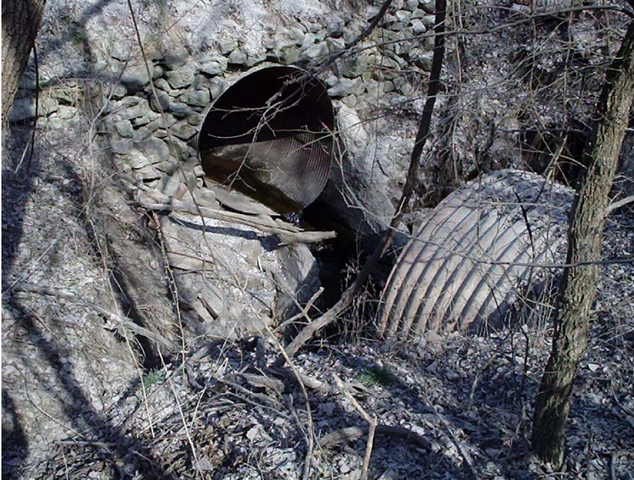
Photo 12D. Missouri River Tributary. Culvert.
