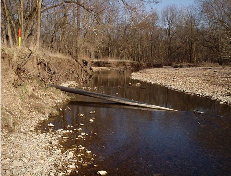
Photo 6C. Clear Creek. Exposed pipe.
